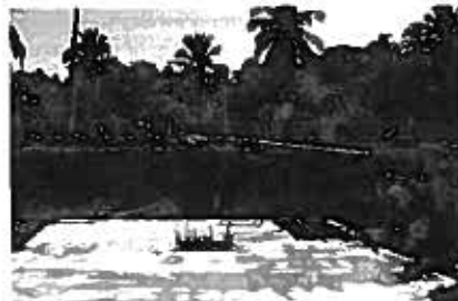
■ A 19,020-gallon capacity septic tank is included in installation
