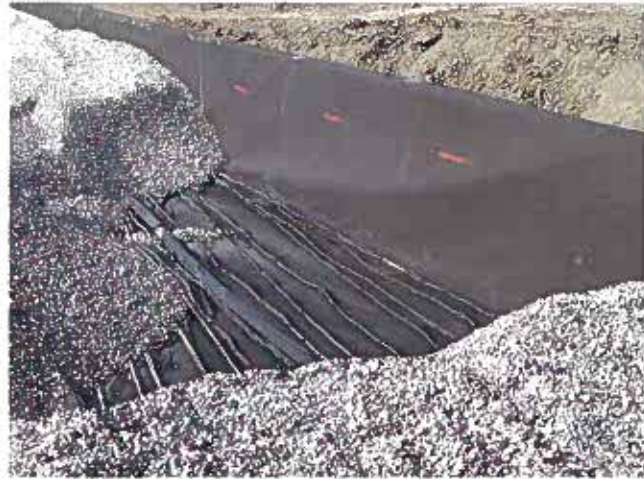
Five feet of technically specified aggregate cover the aeration and underdrain lines.
