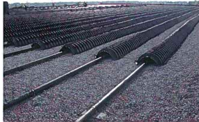
Infiltrator chambers were used at the Buffalo Niagara International Airport as an infiltration bed. The beds uniformly distribute stormwater through the gravel to a system of underdrains.
