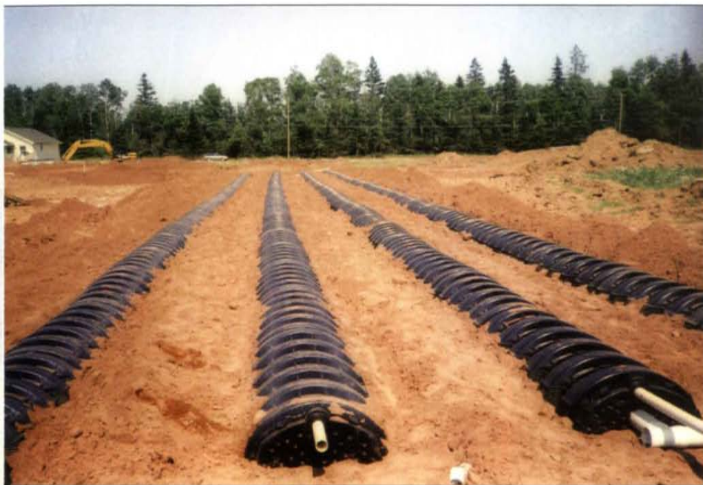
A pressurized Infiltrator leaching chamber disposal field is constructed in a raised bed of sandy fill for the Brudenell Chalets. Each dispersal field zone has four lines that are 150 feet long.
