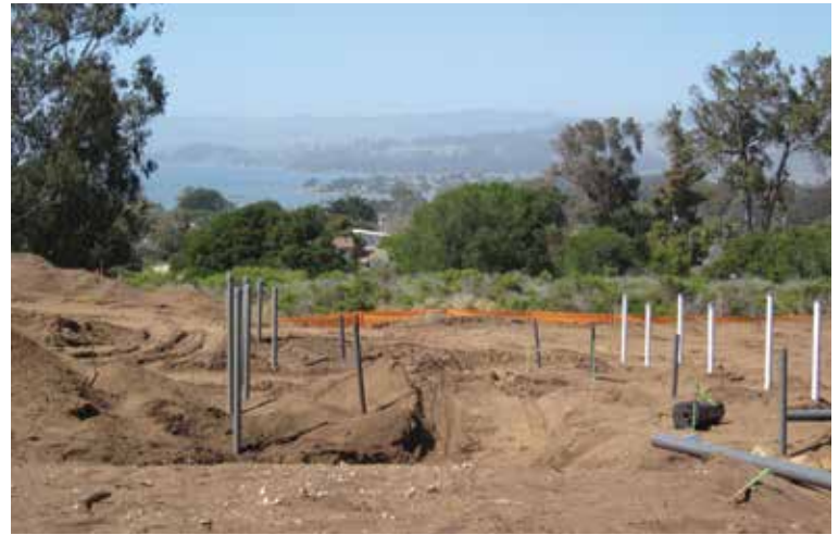
The disposal field is located on a hill overlooking the bay and will provide much needed recharge to counteract saltwater intrusion.
