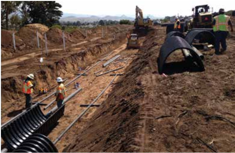
Construction of the disposal and recharge system was fast and efficient. As one crew excavates, another crew installs piping, followed by a crew installing the chambers.
