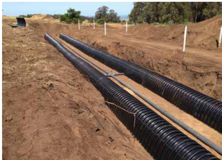
Infiltrator Chambers installed in a trench system offer large volumes of storage to meet peak flow demands.
